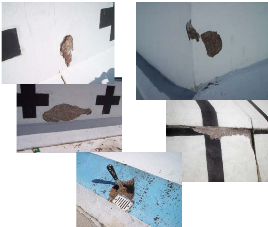
Evidence of deteriorating concrete surface due to continuous finish maintenance and joint deterioration
